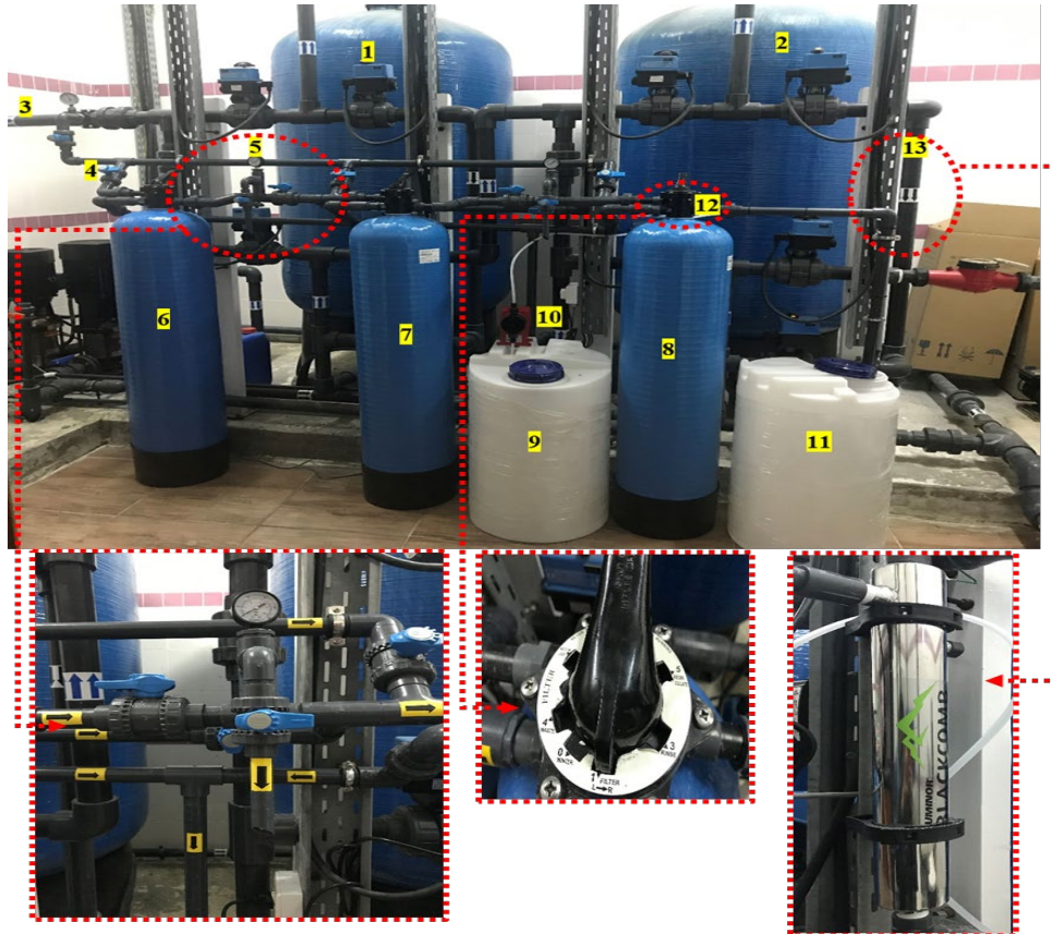
Figure 3.4: Experimental setup showing (1) Existing filter media vessel (2) Existing AC vessel (3) Bypass pipe (4) PVC flow valve (5) Pressure gauge and sampling point (6) Filter media vessel for this study (7) AC vessel for this study (8) GBFS vessel (9) Sodium hypochlorite storage tank (10) Dosing pump (11) Treated water storage container (12) Multi-purpose valve (13) UV unit.
