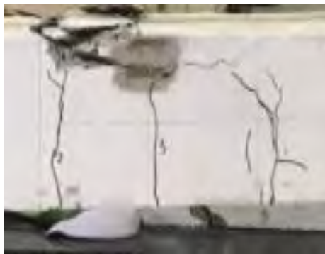
Figure 52: Failure mode of beam 2G10EC.
