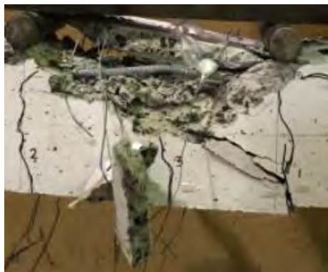
Figure 65: Failure mode of beam 3B10EC.
