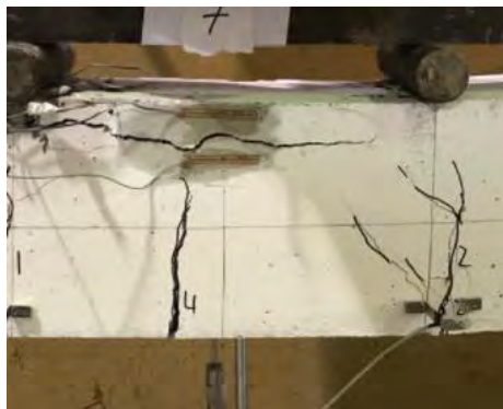
Figure 57: Failure mode of beam 2G10ER.
