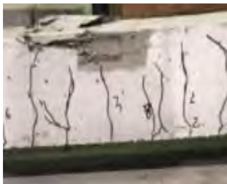
Figure 70: Failure mode of beam 2B10UC.
