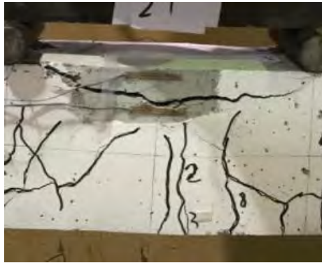
Figure 71: Failure mode of beam 2B12UC.
