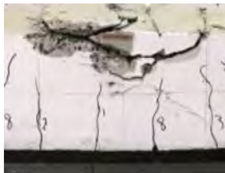
Figure 54: Failure mode of beam 2G20EC.
