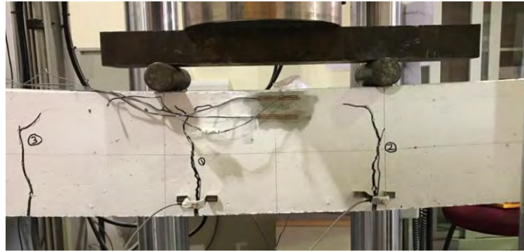
Figure 74: Cracks propagation of beam 2G8EC.
