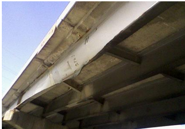
Fig. 1.1: Typical damage in a steel girder due to over-height truck impact [1]
