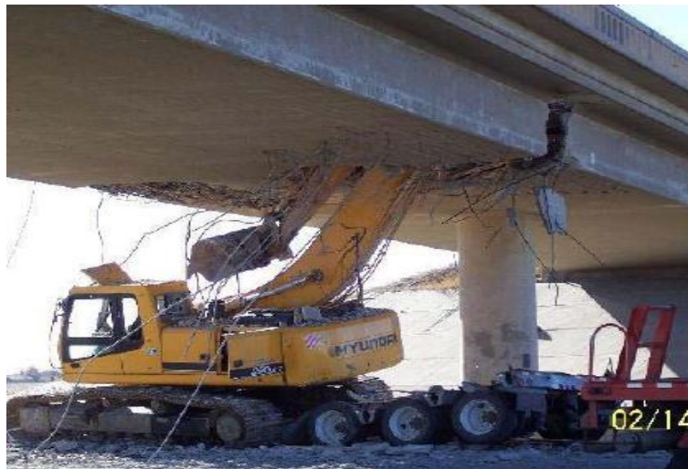
Fig. 1.4: Example of severe damage of a bridge [3]
