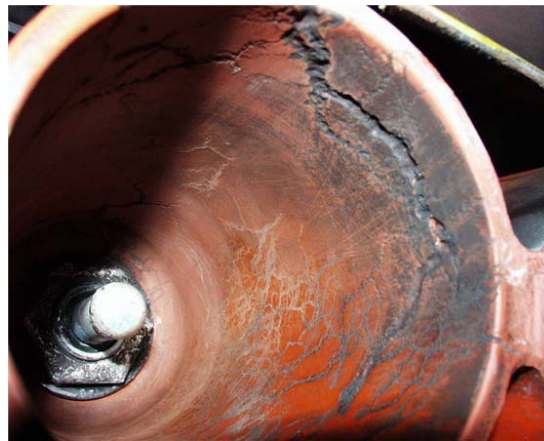
Figure 1: Surface discharge tracking within a cast resin circuit breaker spout [17]
