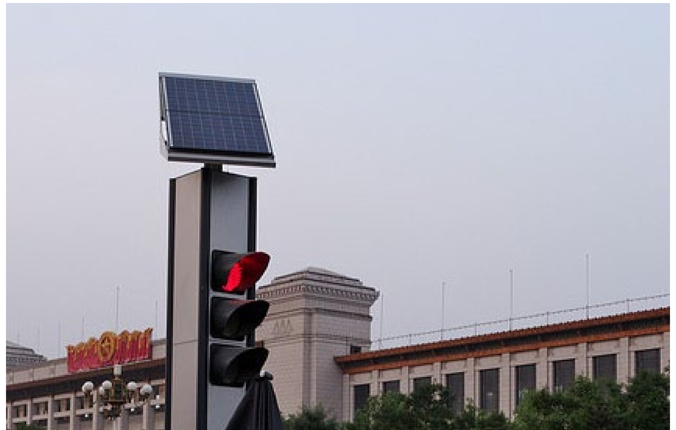
[1] Figure 2: Solar panels in traffic signals
