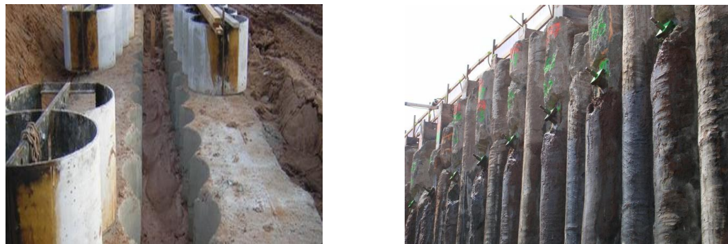
Figure 3. Examples of (a) Secant pile forms, and (b) Secant piles with ties
