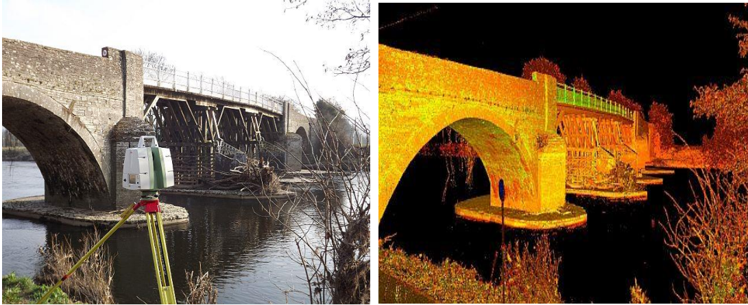
Figure 4: Left: Whitney Toll Bridge, Right: Whitney Toll Bridge laser scanned point clouds [30]
