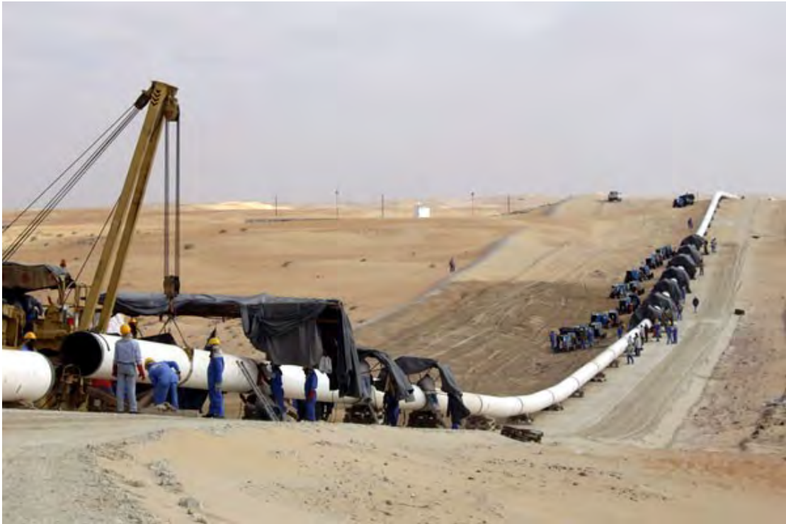
Figure 1: Bu Hasa - Habshan gas pipeline, Abu Dhabi, UAE [11].
