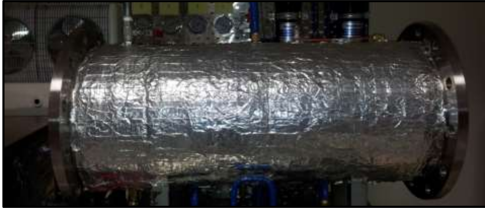
Figure 18: Picture view of thermal energy storage tank
