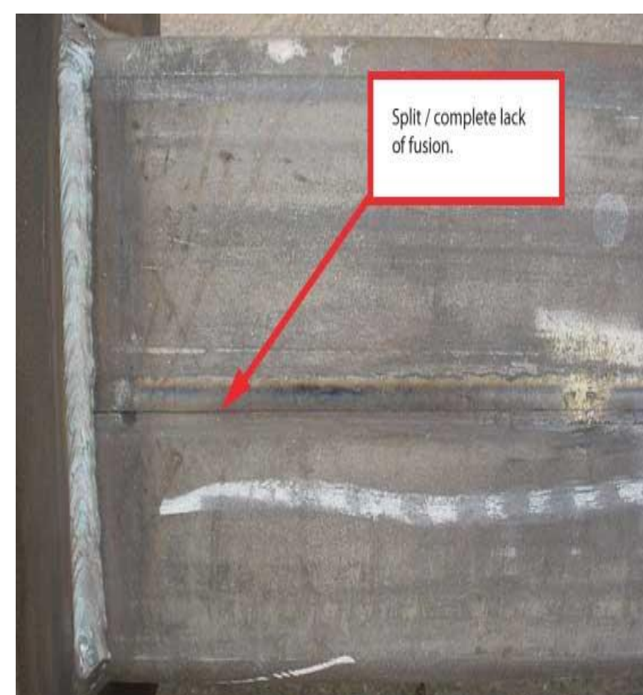
Figure 1: Improper welding of a pipe [3].
