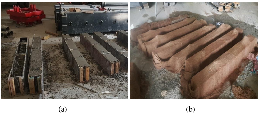
Figure 10: (a) casting process of specimens, (b) curing process of the concrete specimens
