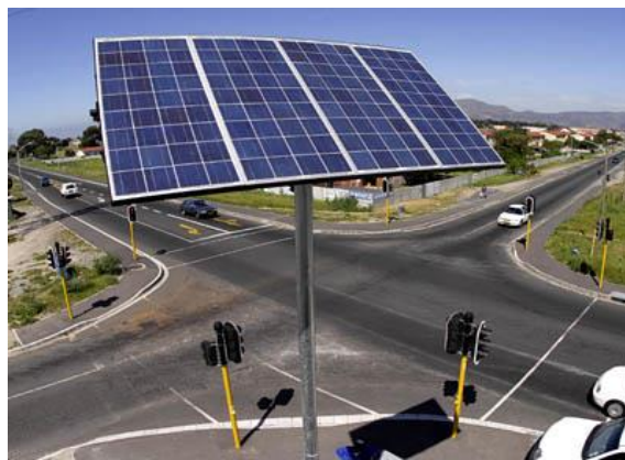
Figure 13 Solar panels powering the traffic signals [67].
