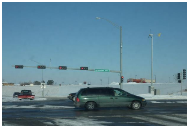
Figure 14 Wind turbine powering the Traffic signals [68].
