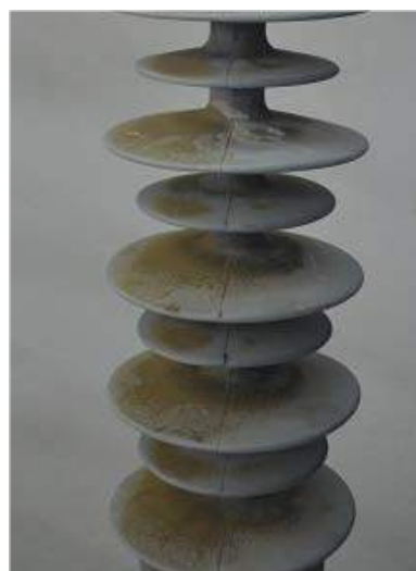
Figure 2.7: Insulator suffering from salt and dirt contamination and discoloration [28].
