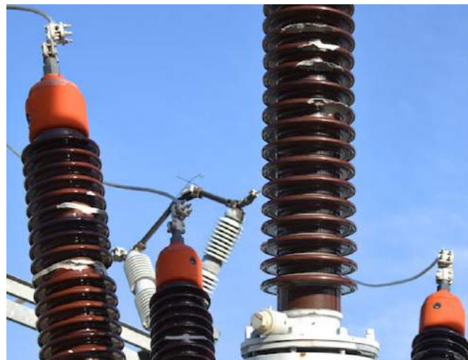
Figure 2.9: Damaged insulators due to vandalism [30].
