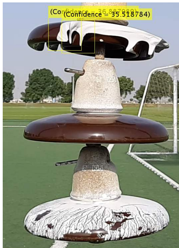
Figure 3.4: Results of AFC object detector for broken insulator inspection.
