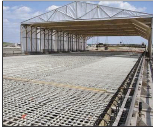
Figure 1: The 18 th street bridge deck reinforced with GFRP bars in Manitoba [10]
