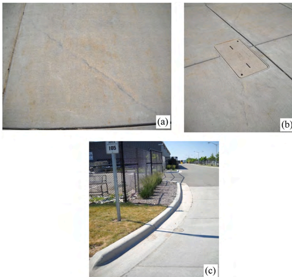
Fig. 17. (a) Cracking caused probably by differential settlement of the flatwork panel; (b) Shrinkage cracking around a rigid insert in concrete; and (c) WG concrete curb at Recycling Center.
