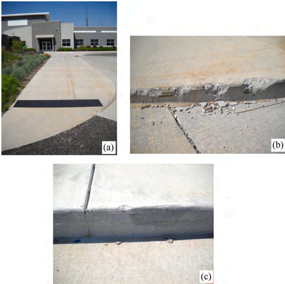
Fig. 16. (a) Sidewalk in front of Recycling Center entrance door; (b) Chipping of the edges of the sidewalk along the road; (c) Control Joint cracks developed in the panels along the road.
